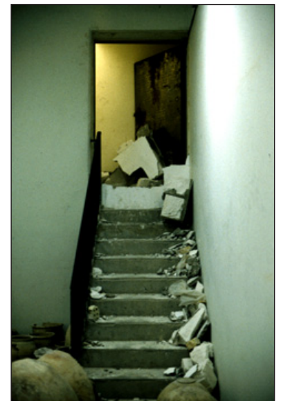
Fig. 23. Basement storerooms, walled-up doorway breached by looters (© J. Russell)
